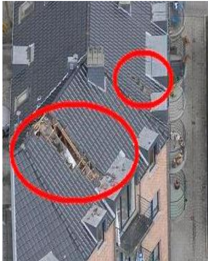
Figure 4: Damage to the roofs.
