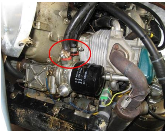
Figure 8: Picture of the rubber pipes as fitted on the connectors on sandwich plate.
