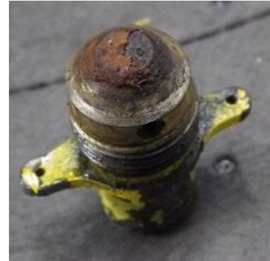
Figure 16: Drain valve of the compensation tank
