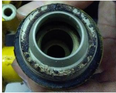
Figure 12: Contamination along the shut off valve seat
